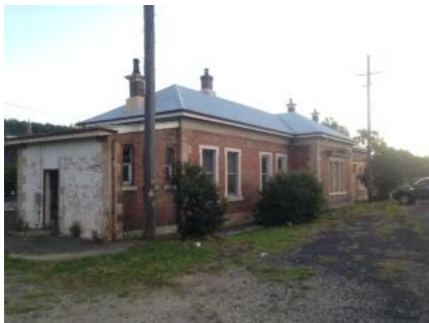
Missing chimney capping (second from left)
