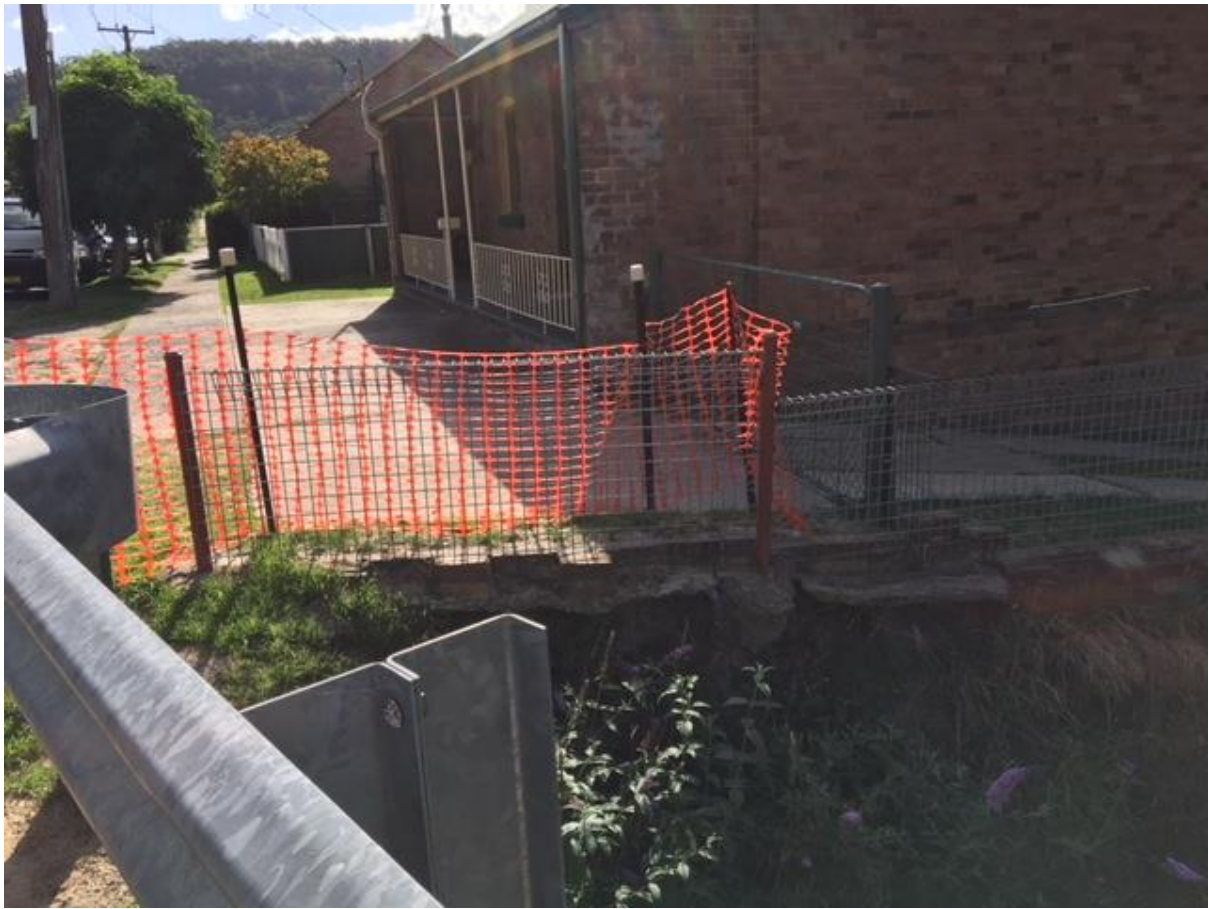
Erosion on Council Road reserve adjacent bridge
