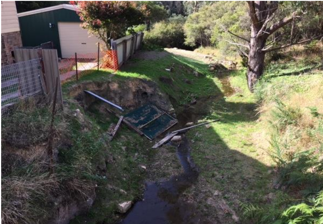
Erosion on Austen & Butta Land. Land owned by Bradford on left.
